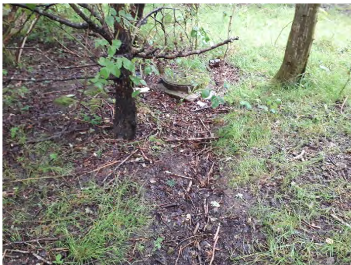
Possible soakaway chamber
