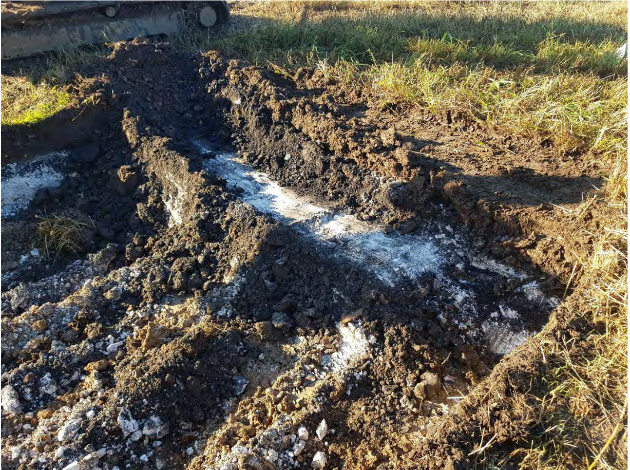
Plate 9 – View of the encountered Made Ground materials
