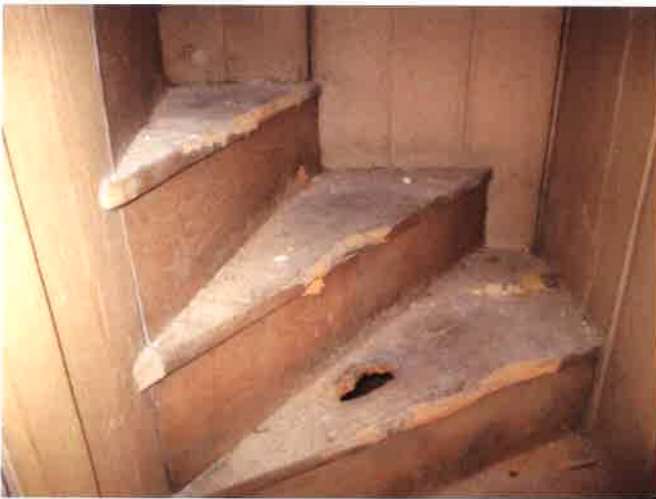
p26 timber decay
