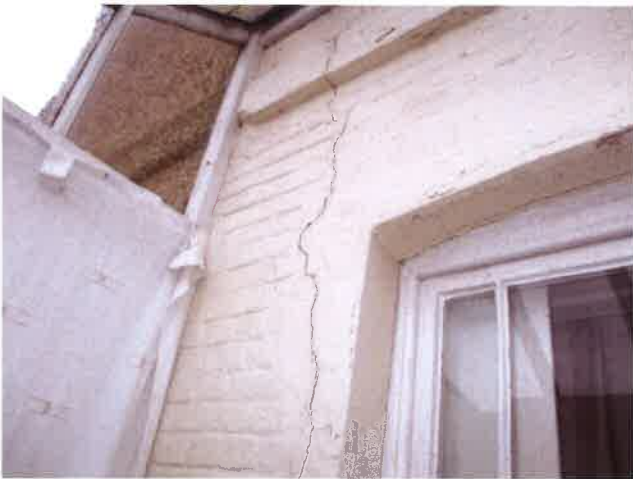
p 37 structural crack
