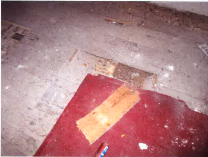
p35 timber decay
