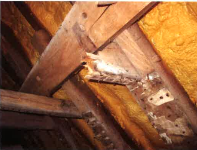
p32 timber decay
