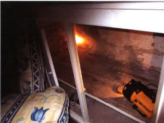
p 21 decayed bricks/ damp
