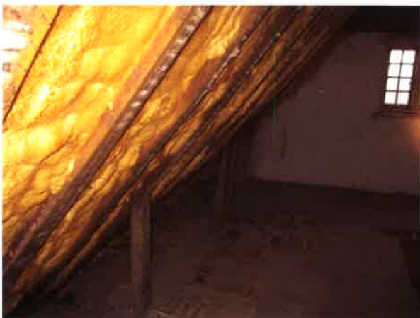
p 34 sagging timbers
