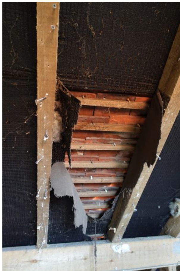
Plate 4: Felt sarking damage
