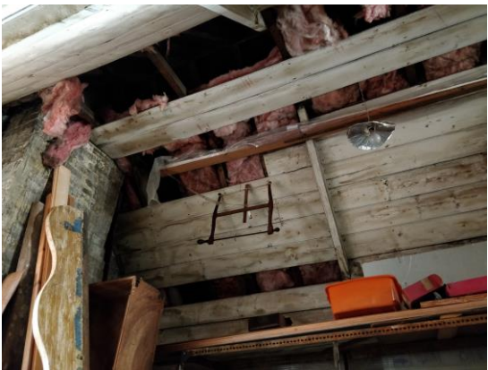
Condition of ceiling to rear section
