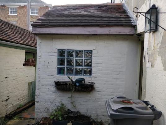
Poor construction of existing utility room.
