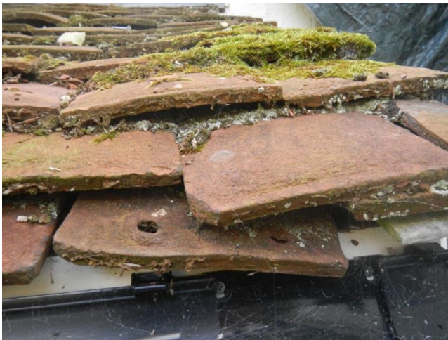
Detail of lifted tile
