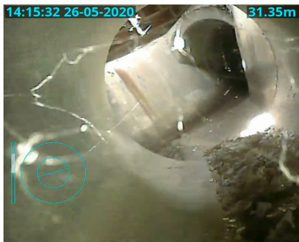
Pipework shows SILTING
