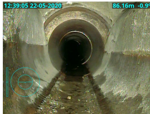
Cracked pipework – still from video
