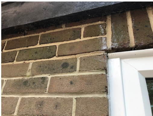
Cracking Adjacent Door
