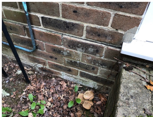
Displaced Brickwork at Low Level
