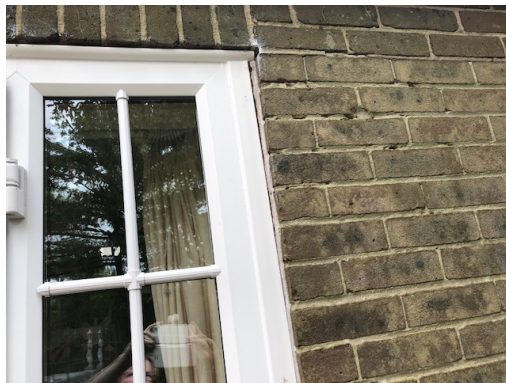
Cracking Adjacent Door
