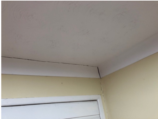
Cracking and Displacement to Ceiling
