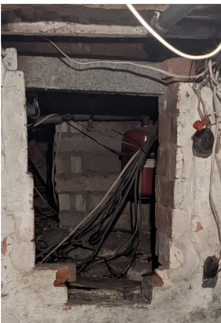
(Photograph 3 – Reduced height void)
