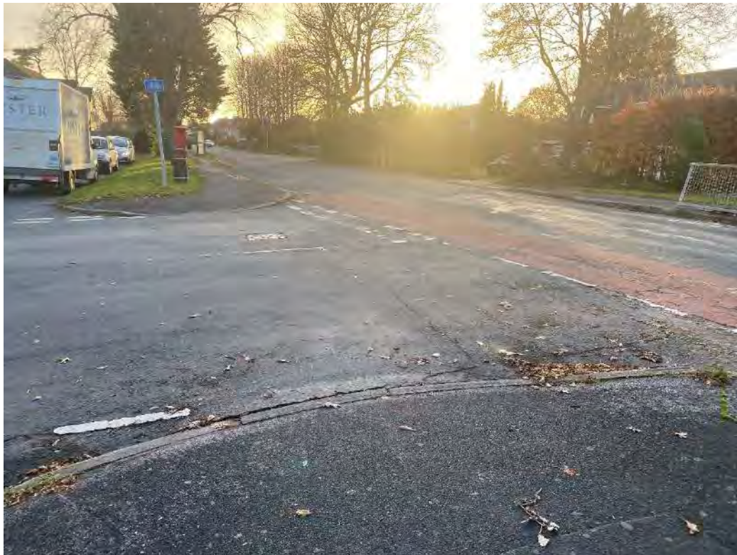
Image 3: Lack of tactile paving at Ward Crescent junction
