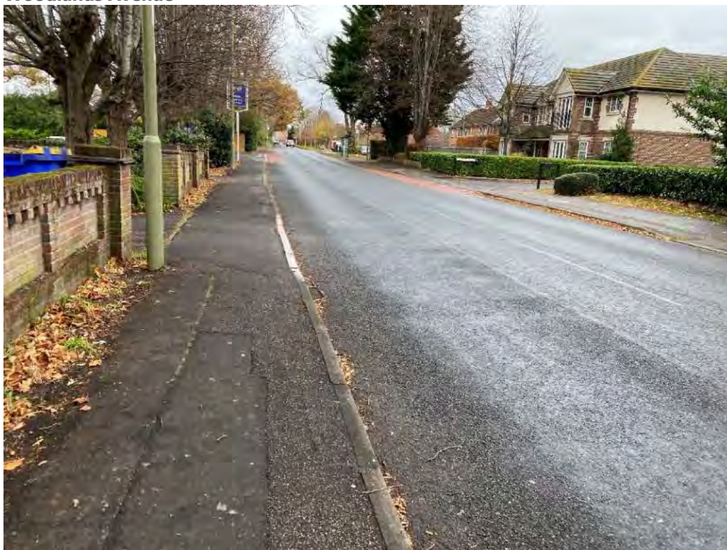
Image 4: Lack of dropped kerbs/tactile paving at Pedestrian link from New Brighton Road to Woodlands Avenue
