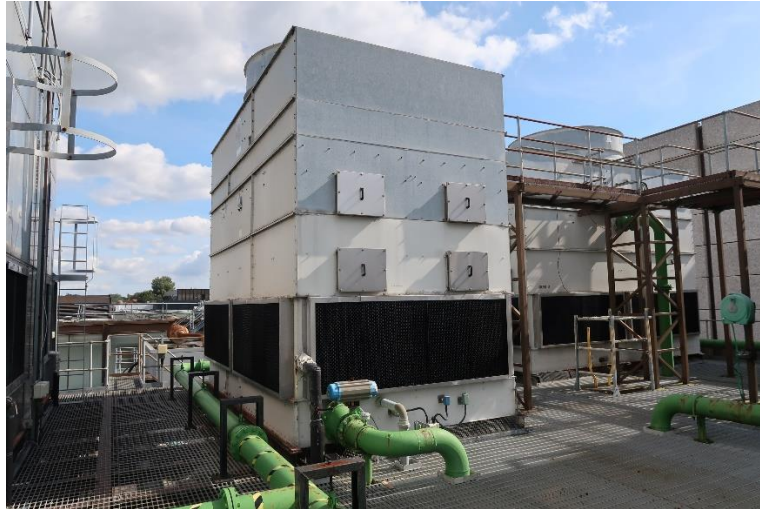
Fig 4.3 - Existing Energy Centre
