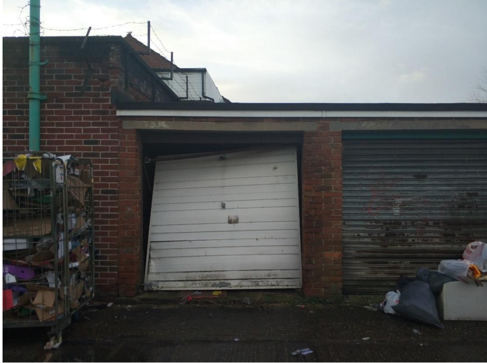
Fig. 9 - Photo showing garage was broken in by thief
