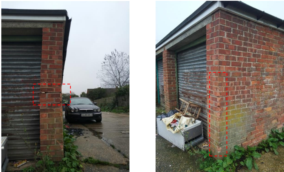
Fig. 13 – Photos showing the damaged existing garage.
