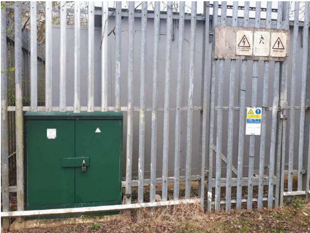
Plate 15: Close up of electric substation and associated infrastructure.
