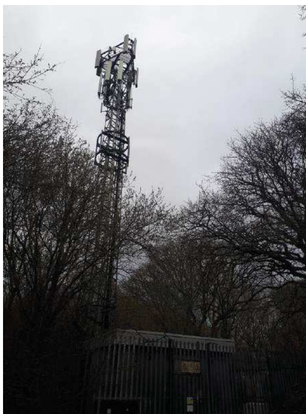
Plate 14: Vodafone telecommunications mast and associated electrical substation.
