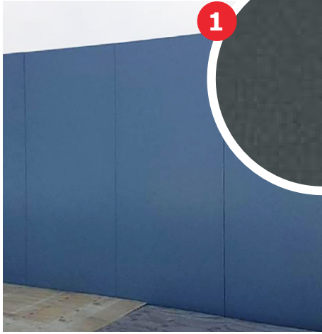
Vertically Laid Roof Plant Screening: Metal Panels in Anthracite RAL 7016 (1)
