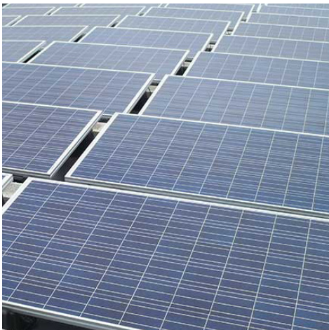
PV Panels: Rooftop Solar Panels
