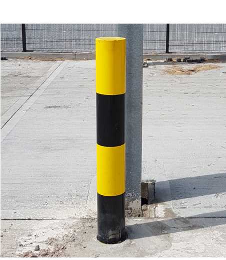
Bollards: Steel PPC in Black & Yellow
