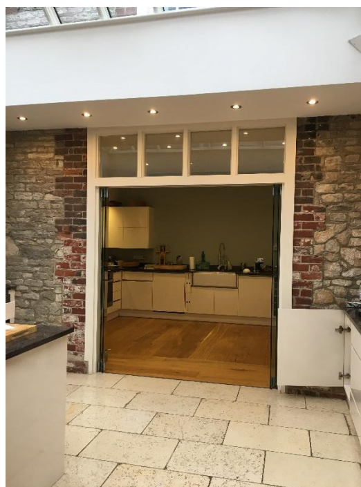
Figure 11 Existing kitchen floor to be replaced with similar stone flooring.
