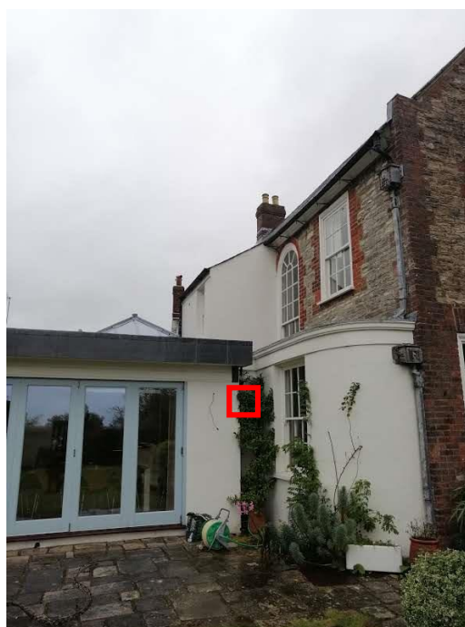
Figure 9, Cast iron extraction grille connected to ground floor WC
