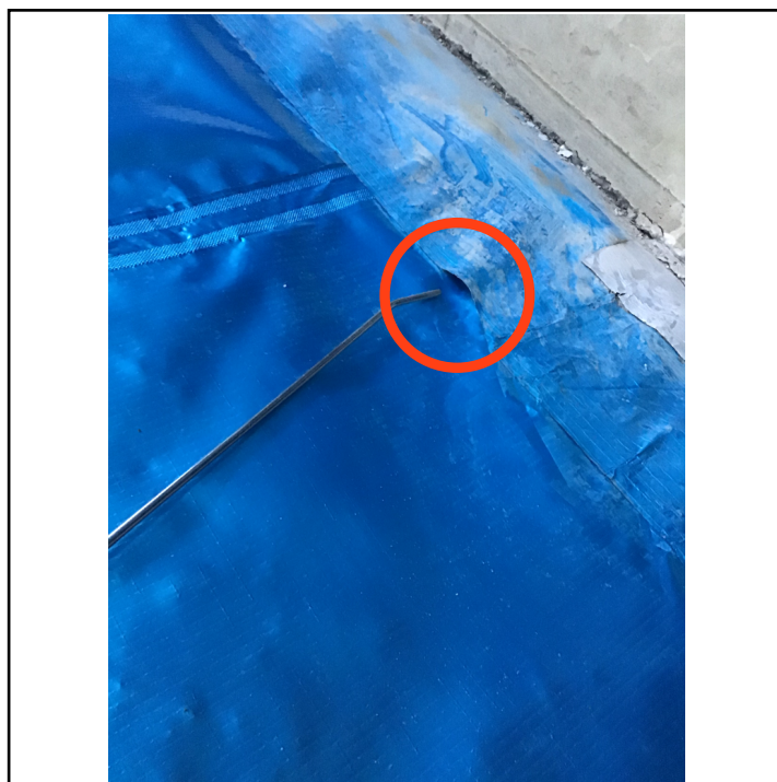
Example of miss-weld fault identified.
