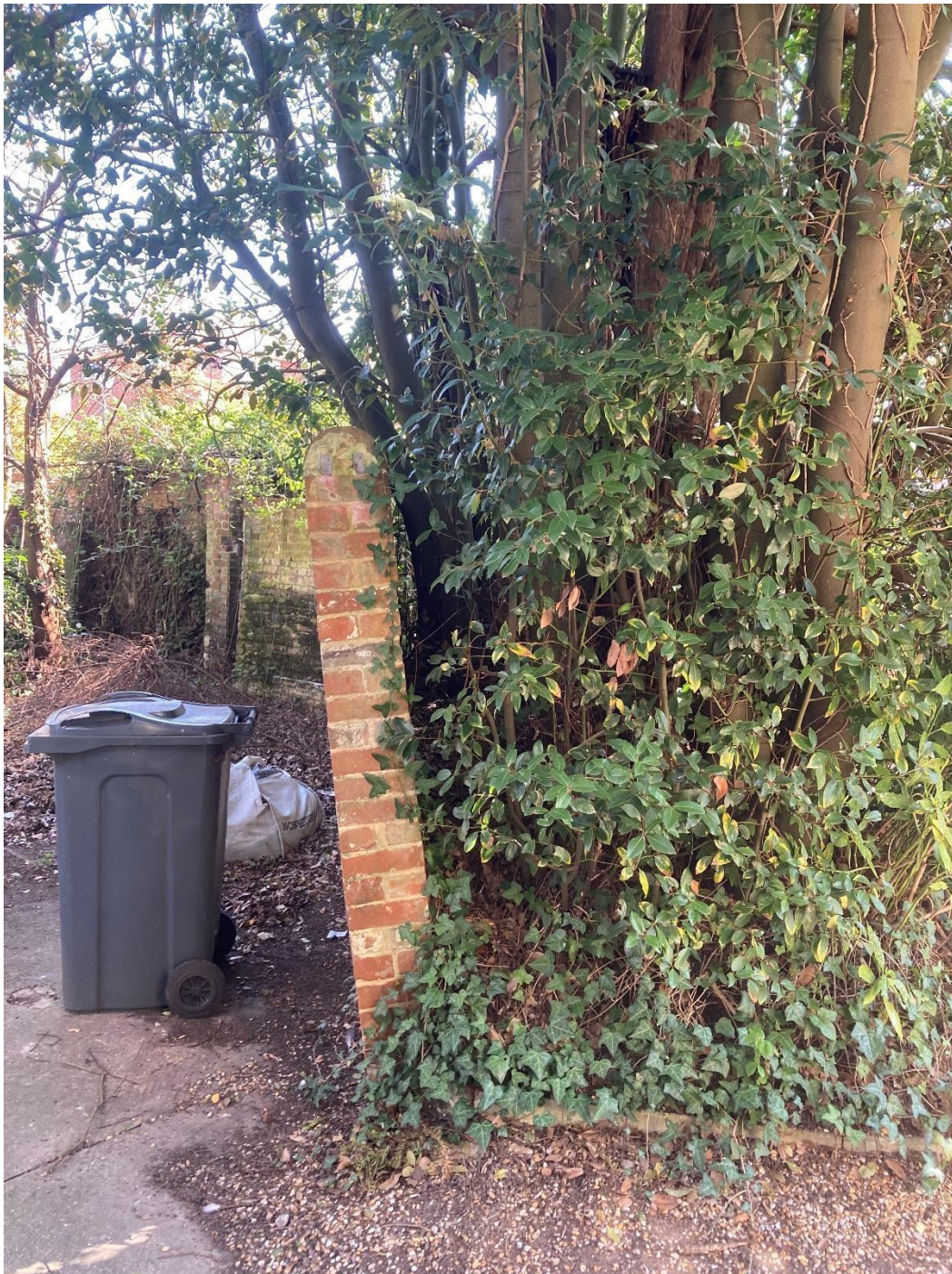
SAL8 Direct damage to adjacent wall from G10 and potentially G11.
