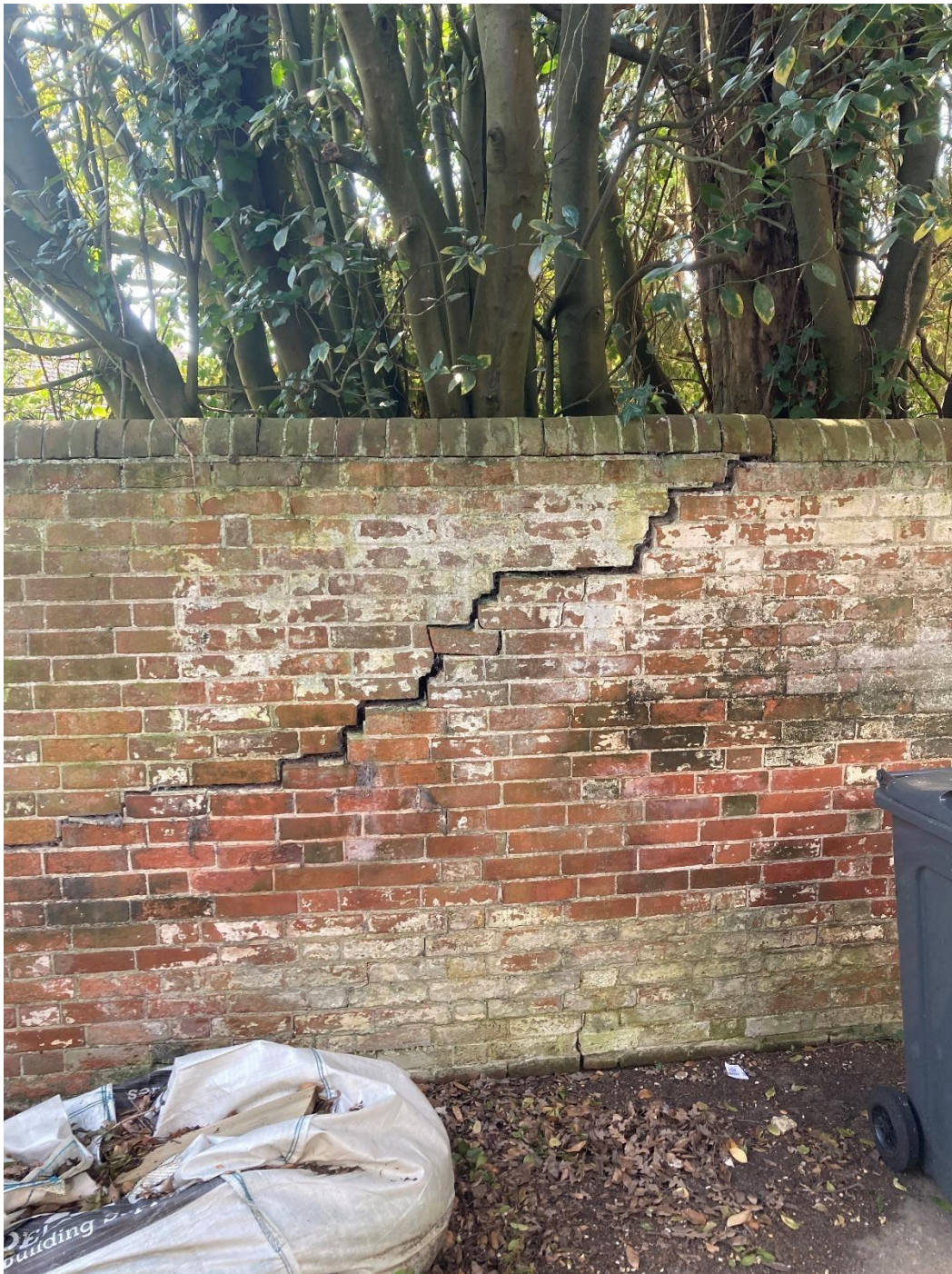
SAL7 Direct damage to adjacent wall from G10 and potentially G11.
