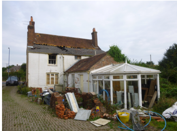
The rear elevation of the dilapidated house that stands on the site.
