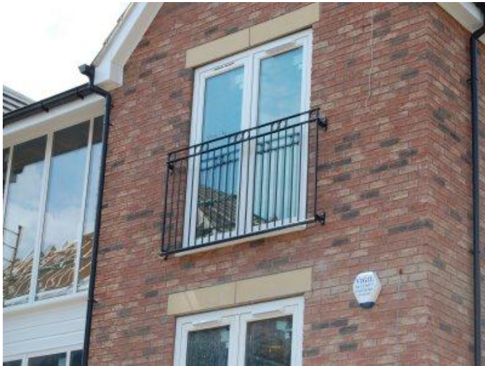
Black UPVC 110mm square guttering and 68mm rainwater downpipes
