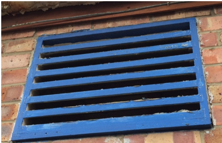
Figure 5. Wooden, unobstructed vent within courtyard area.
