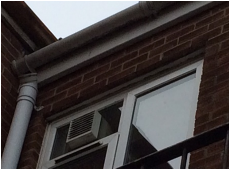
Figure 4. Gaps underneath fascia along the roofline within the courtyard area.
