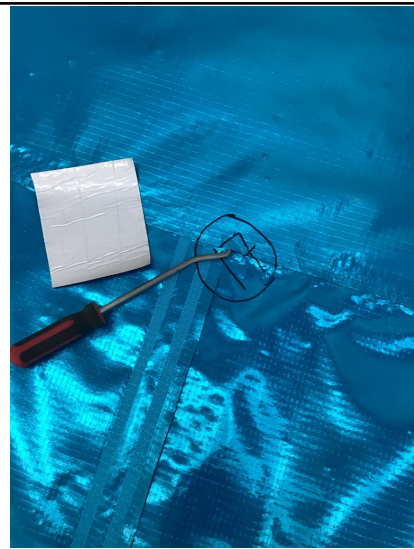
Fault found within the T-section of the membrane.
