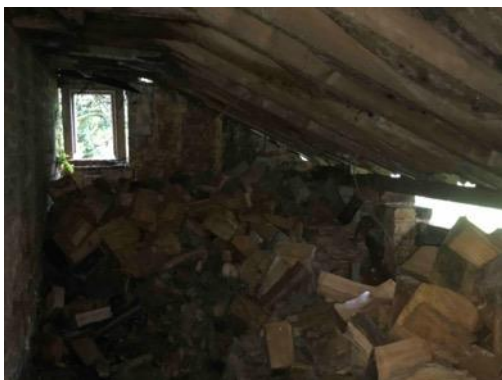
Photo 29: Internal view of log store showing daylight visible at eaves level. B7.
