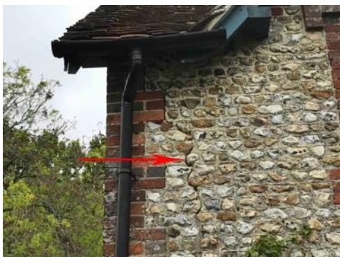
Photo 33: Crack in stonework of south-facing elevation.
