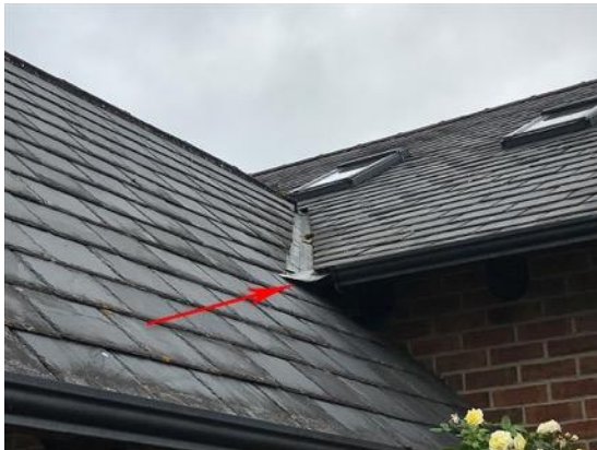
Photo 5: Red arrow points to gap leading beneath lead flashing at hipped joint.
