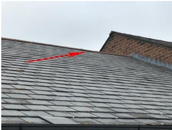
Photo 3: Red arrow points to gap leading beneath ridge capping. Single-storey element.
