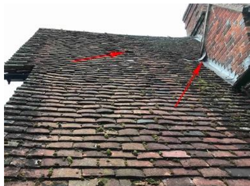
Photo 34: Gaps leading beneath lead flashing and raised clay roof tile. North-facing elevation.
