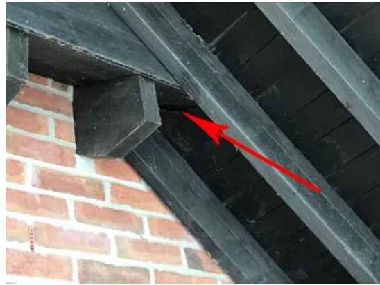
Photo 6: Red arrow points to opening leading to cavity within timber porch. Front south-facing elevation.
