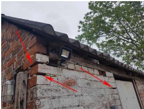
Photo 14: Red arrows point to cavities caused by failed mortar within brickwork. B3.
