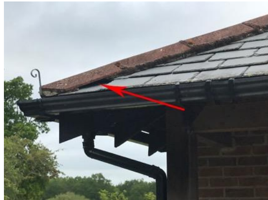
Photo 4: Red arrow points to gap leading beneath ridge-capping caused by failed mortar. Single-storey element.
