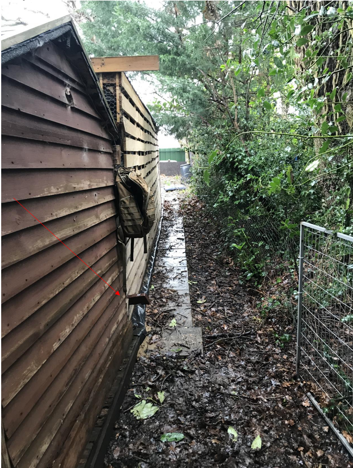
Photo 3. Rainwater outlet marked with an arrow
