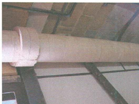
Vicutube in main switch room
