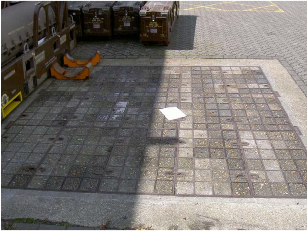
Photograph 3: Location of UST
