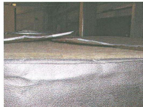
Encased Rockwool on main air distribution duct
