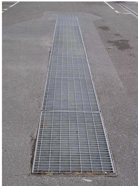
Photograph 2: Overflow storm drain
