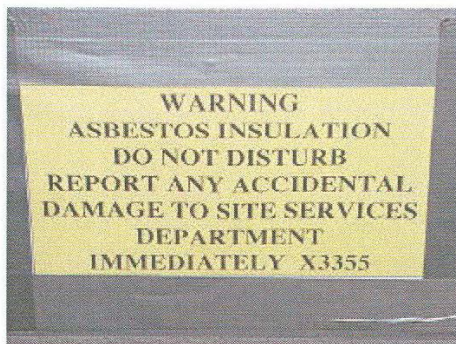
Warning sign adjacent restaurant boilers
