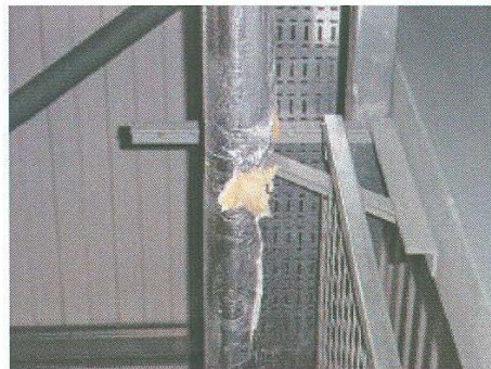
Rockwool lagging on pipes
