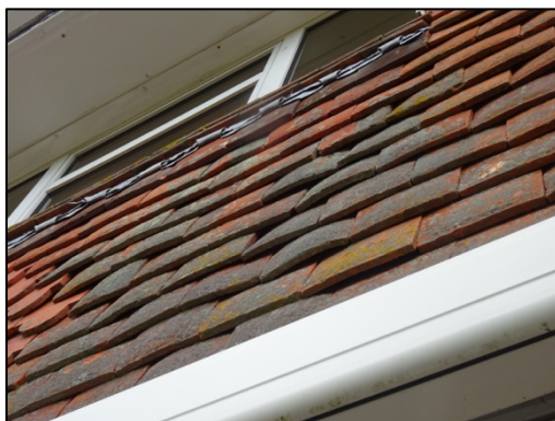
Figure 8 – lifted hanging tiles on the western elevation of the house
