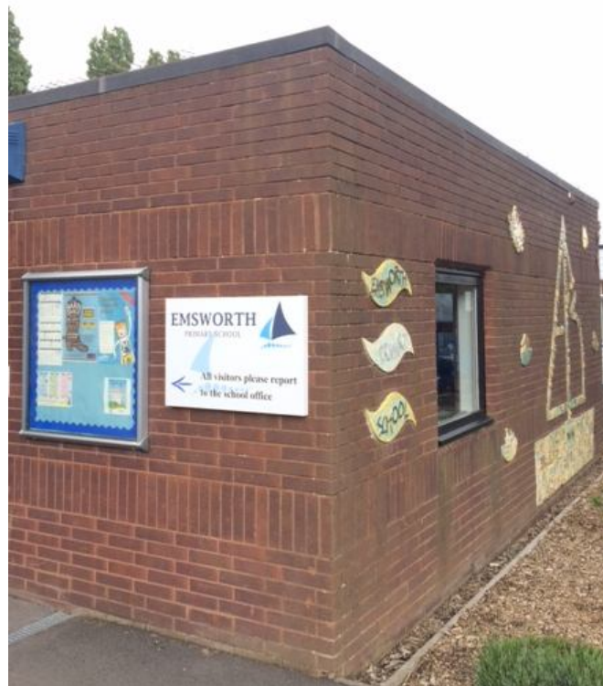
Figure 3: Main entrance to Emsworth Primary School displaying SCOLA building and slight gap between roofing material and brickwork.
