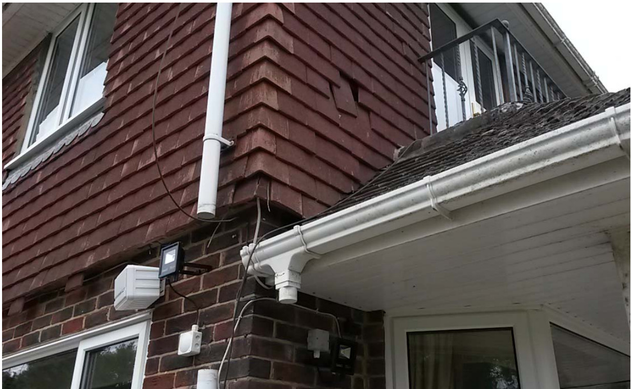
Photograph No. 08 - Potential access point noted where 1 no. hanging tile was missing. No evidence of bats using this point was noted.
