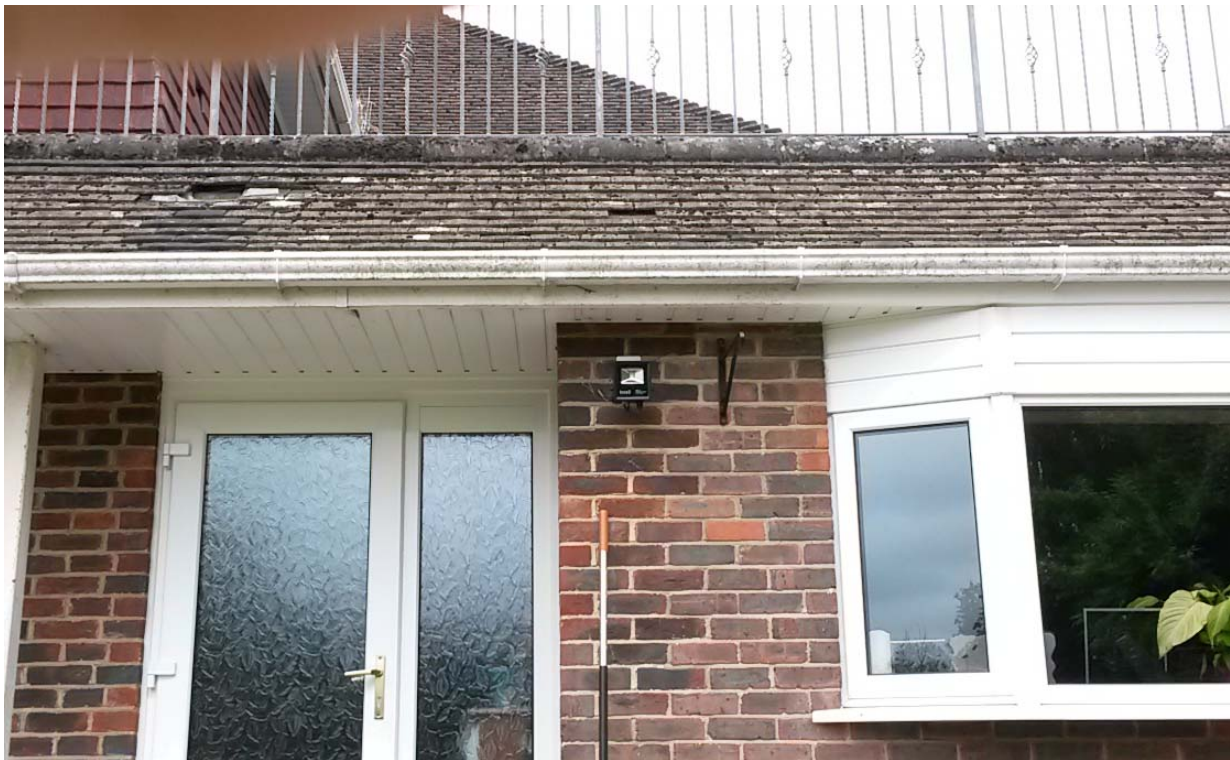
Photograph No. 06 - Potential access point noted where 1 no. roof tile was missing. No evidence of bats using this point was noted.
