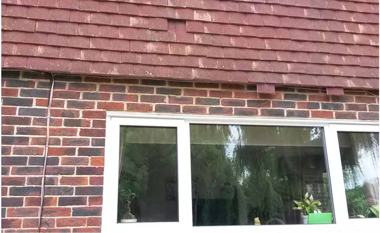
Photograph No. 07 - Potential access point noted where 1 no. hanging tile was missing. No evidence of bats using this point was noted.
