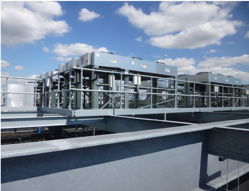
View from roof level of existing Liebert MCL Condenser units
