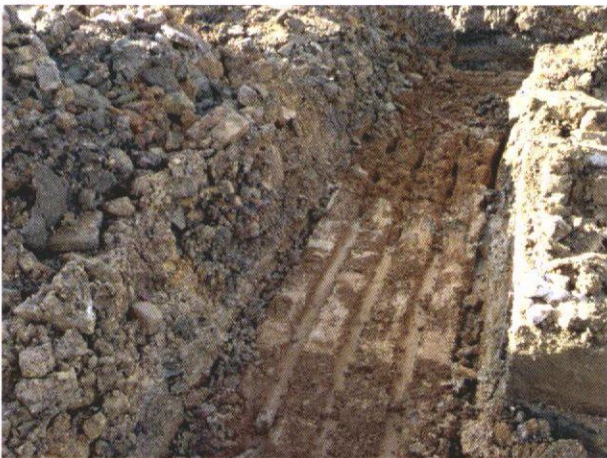
Photograph showing the southern side of the tank base - note the limited relic oil stained clay to 0.25m
