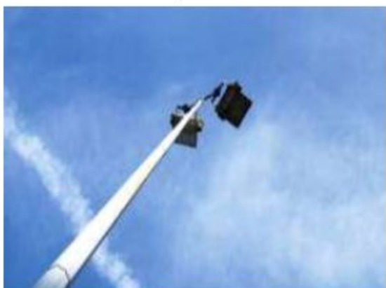
Example of 12m high floodlight
