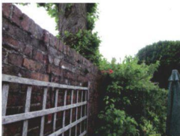
View along wall on neighbours side – shows wall leaning 70mm at top
