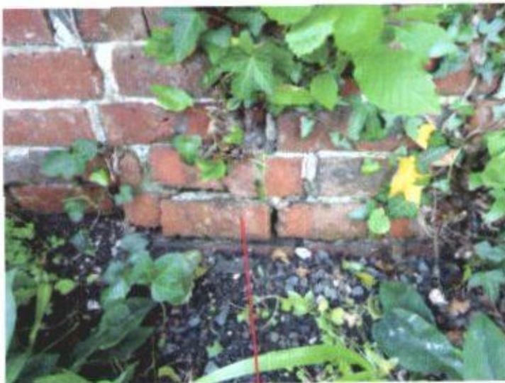
Damage to base of wall (neighbours side)
