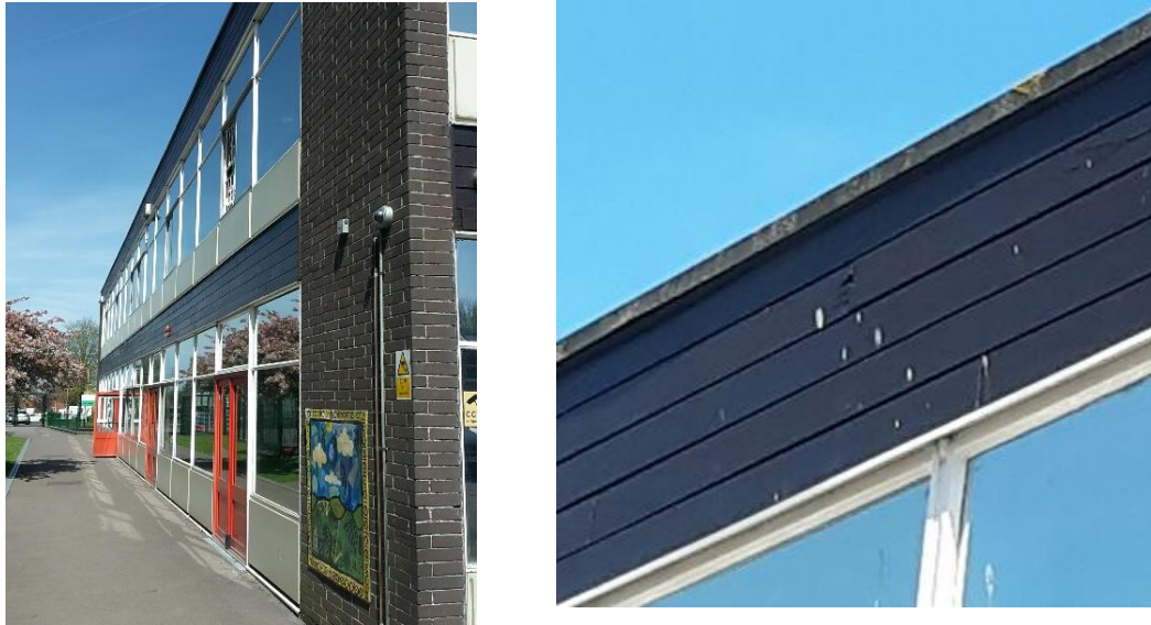
Figure 3: Photographs of the building. Above right shows gap in cladding identified on the west of the building
