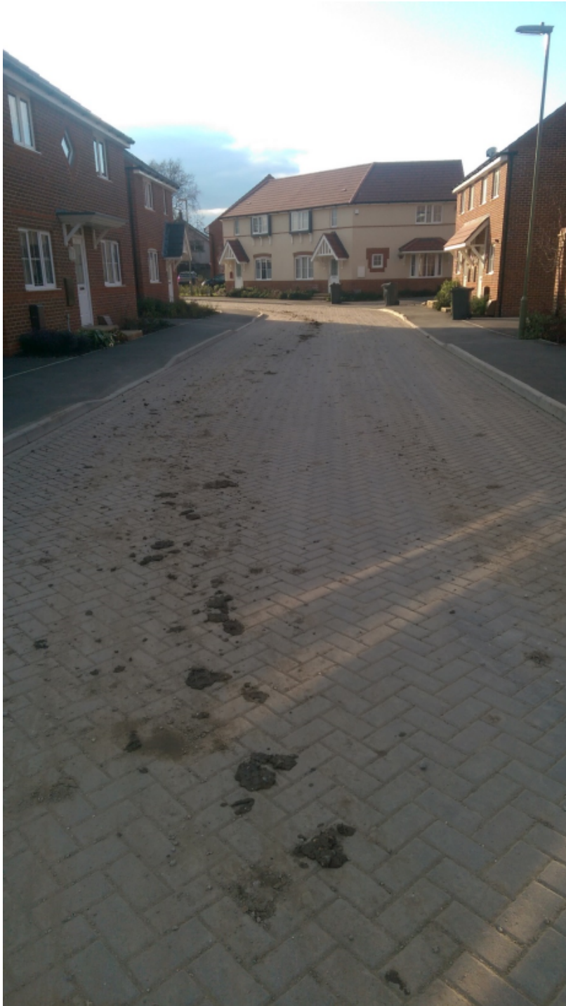
Image No.10 – Permeable paving on Copsey Nursery being used by construction traffic causing blockage of the joints
