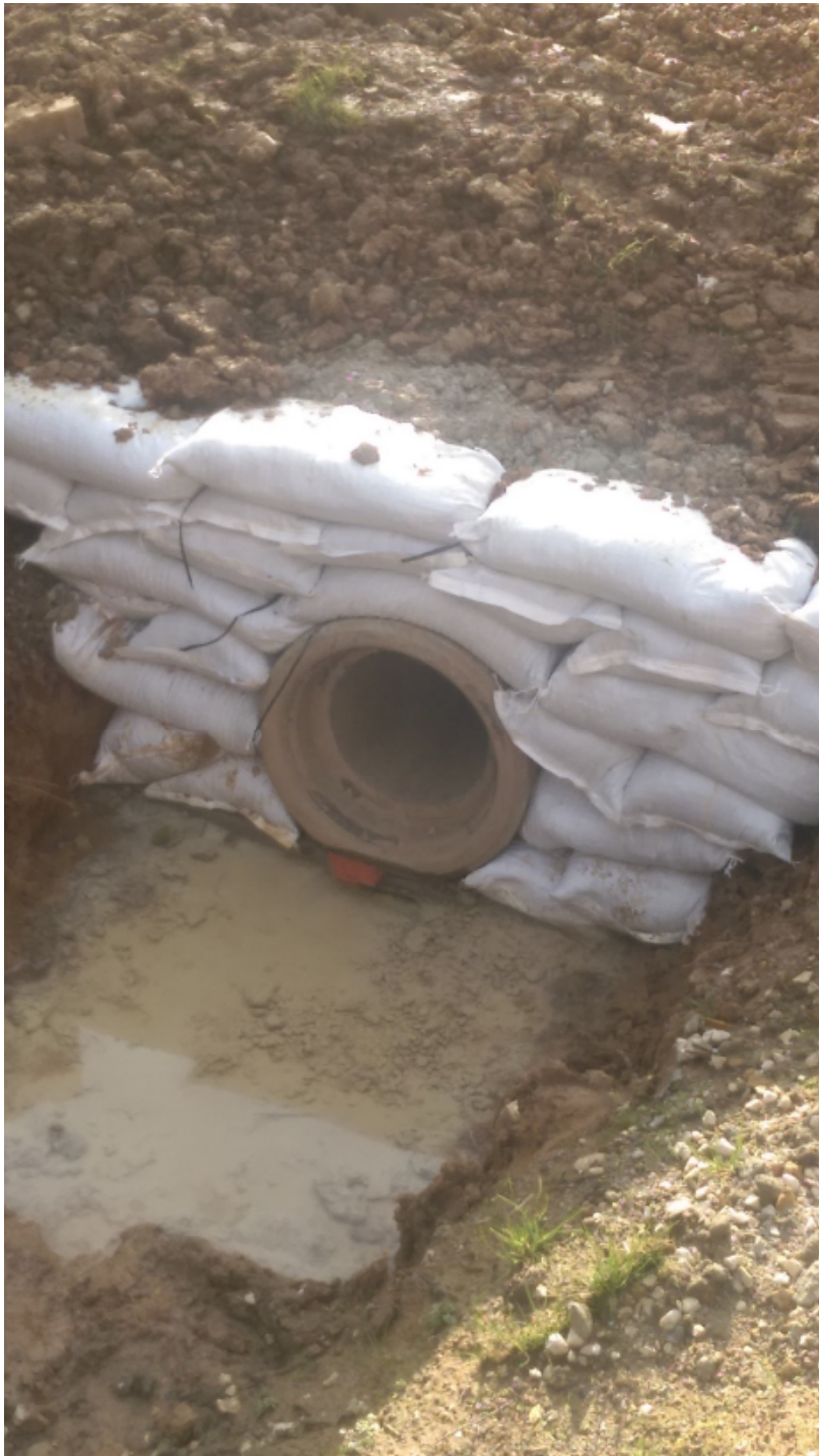
Image No.7- Copsey Nursery land drainage outfall
