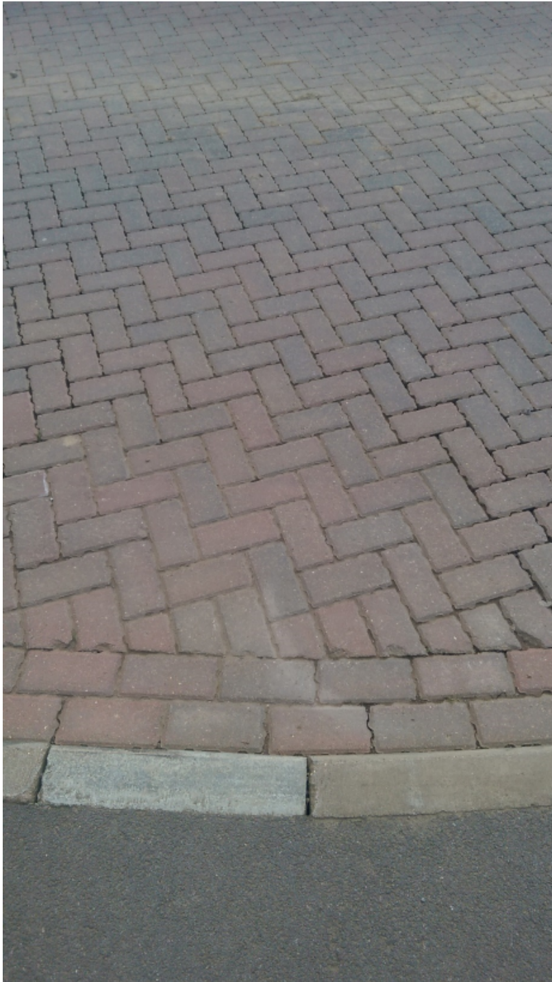
Image No.9 – Permeable paving in Copsey Nursery with evidence of ponding due to infilled joints
