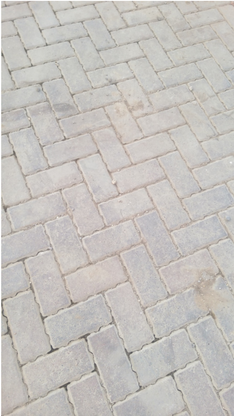
Image No.8 – Permeable paving in Manor Farm with evidence of joints infilled with mud
