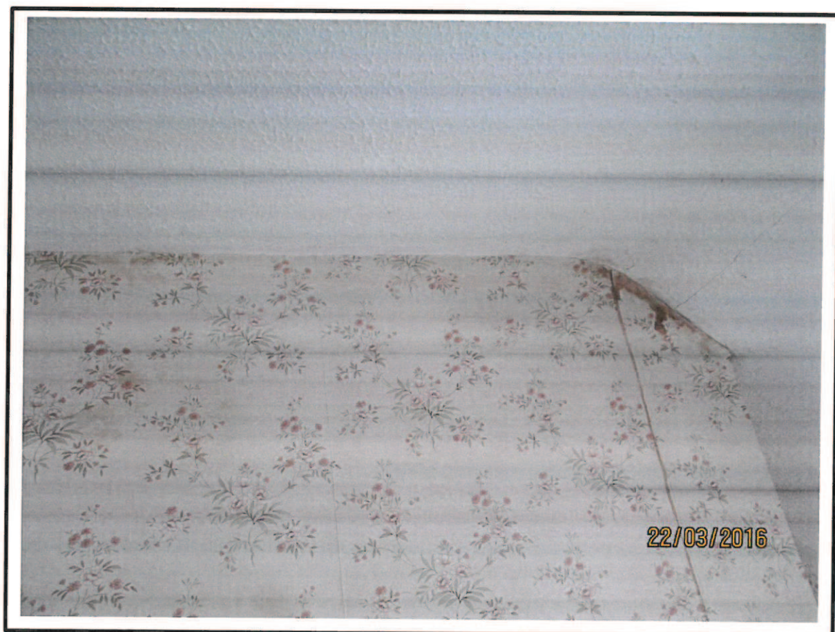
Staining to chimney breast
