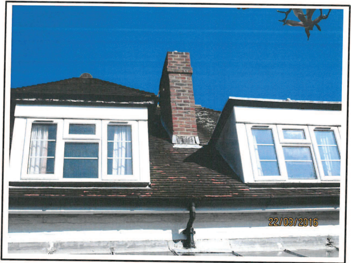
Chimney and delaminating tiles
