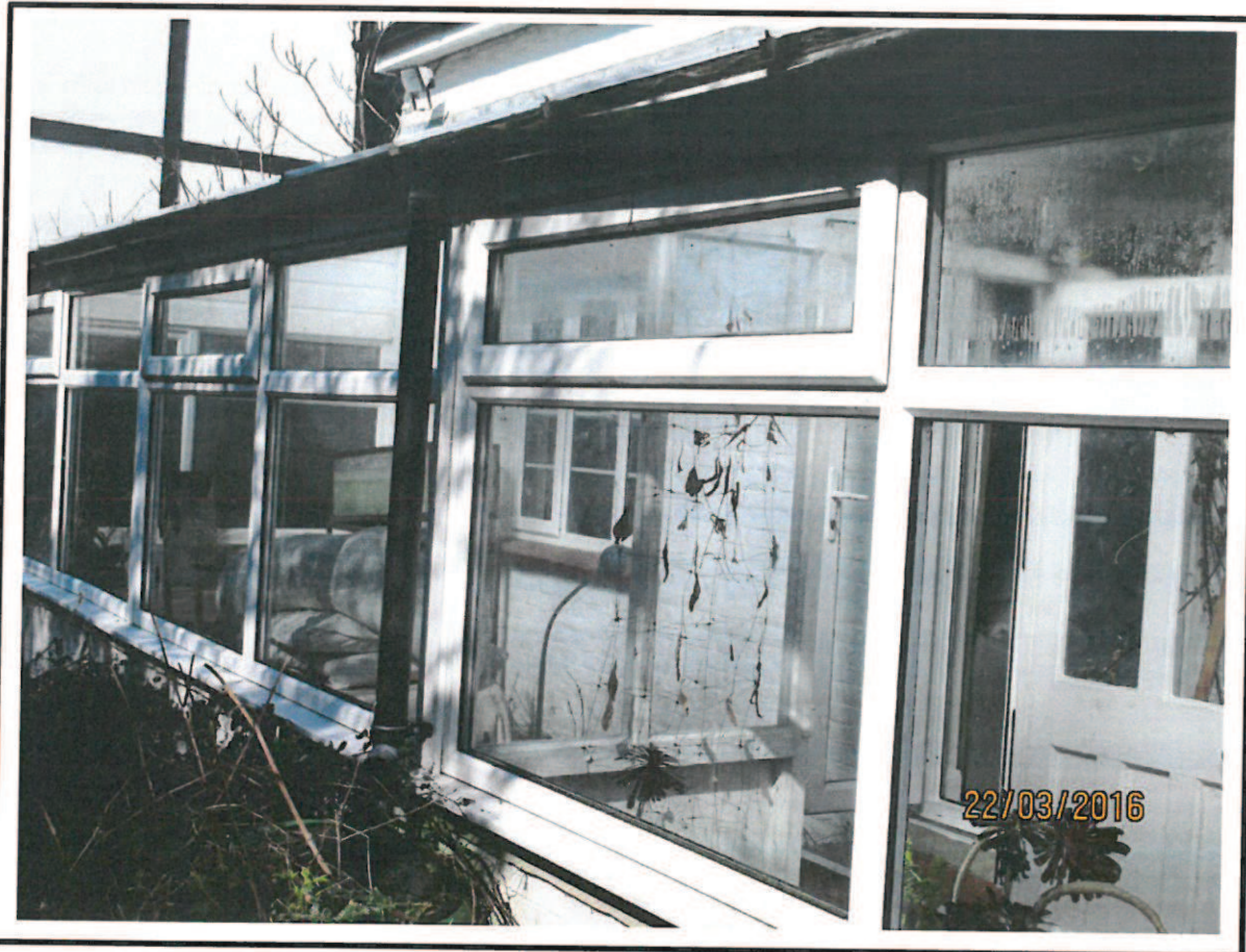
Distorted gutter to rear conservatory
