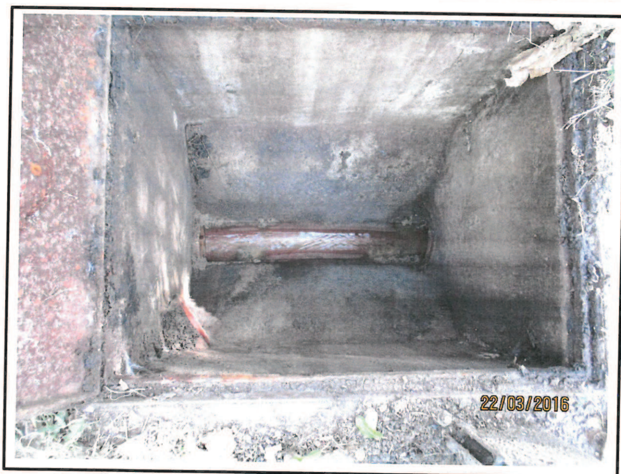
Middle drainage chamber
