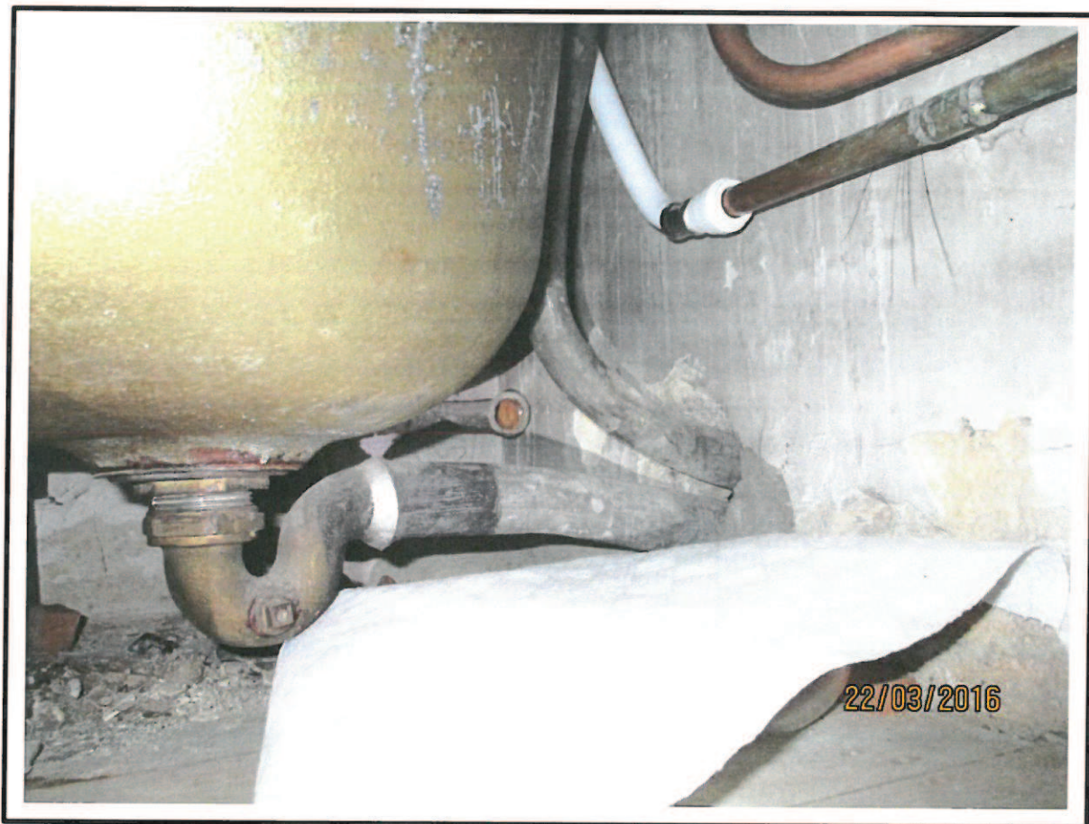
Lead wastes to bath
