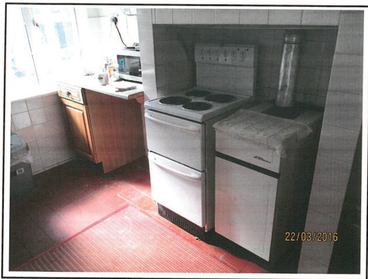
Boiler in chimney recess
