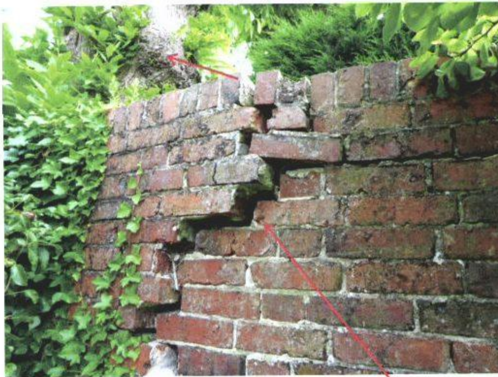
View from neighbours side – Wall leans 70mm at top – wall is unsafe
