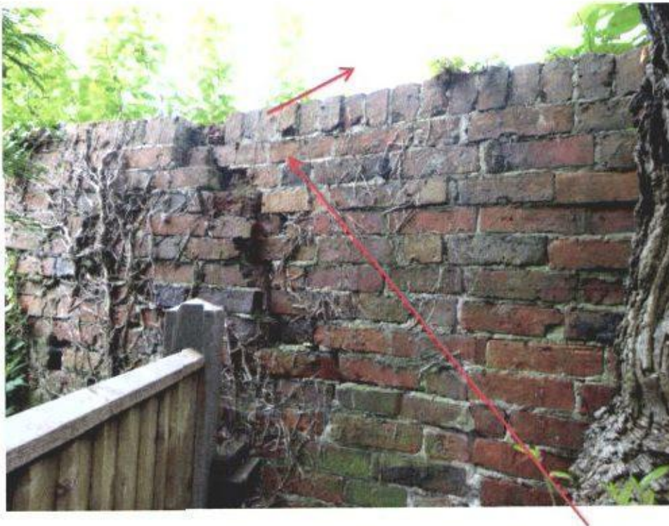
Left hand corner behind tree – wall has been pushed over 70mm at top
