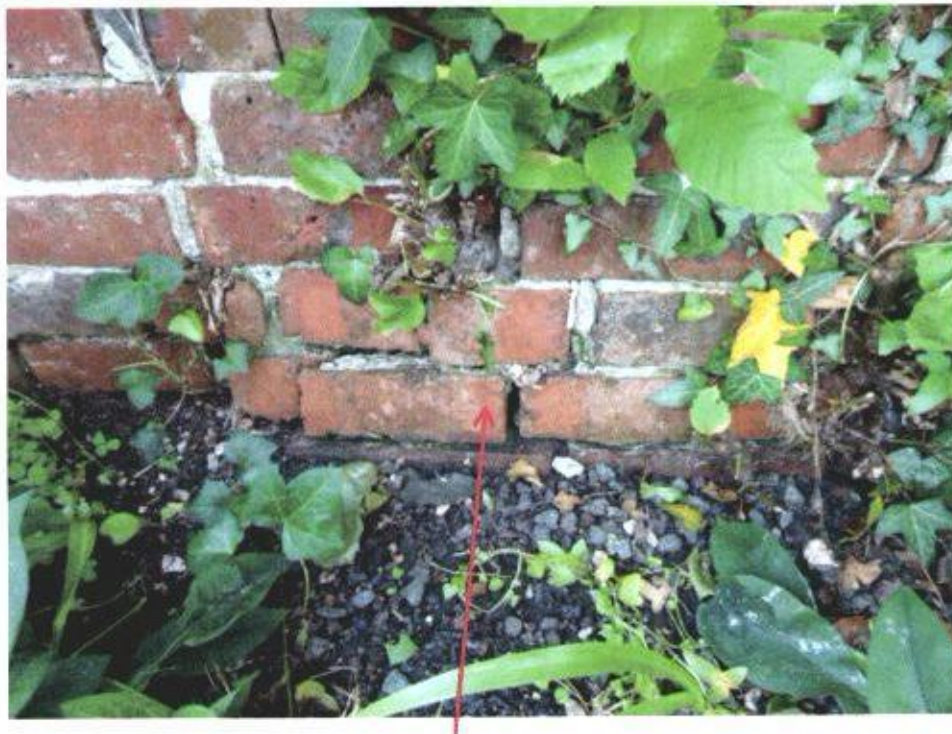
Damage to base of wall (neighbours side)
