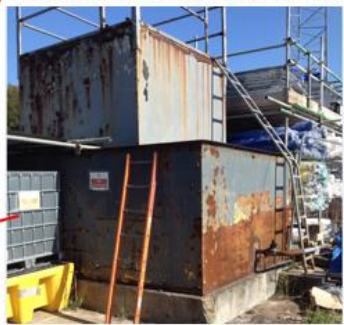
Above ground mounted tank to the North of the garage
