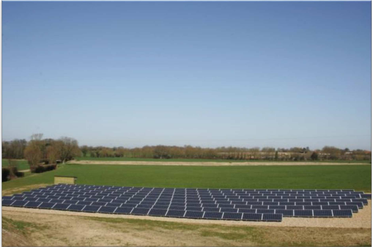
Figure 5 – Example of PV array using similar mounting system
