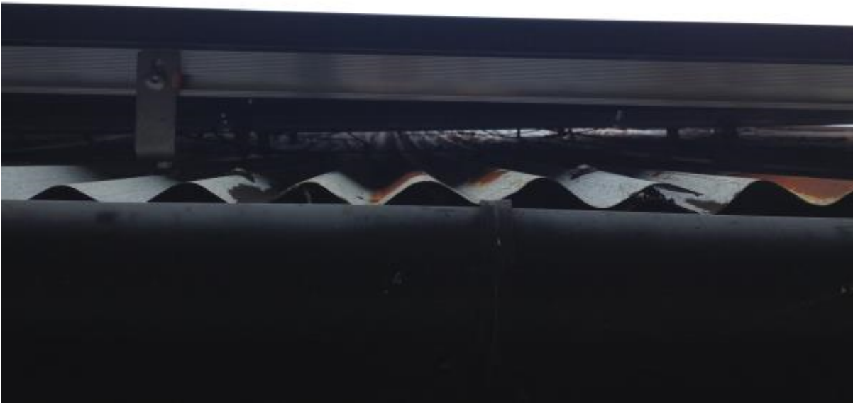
View of solar panels and connection to roof
