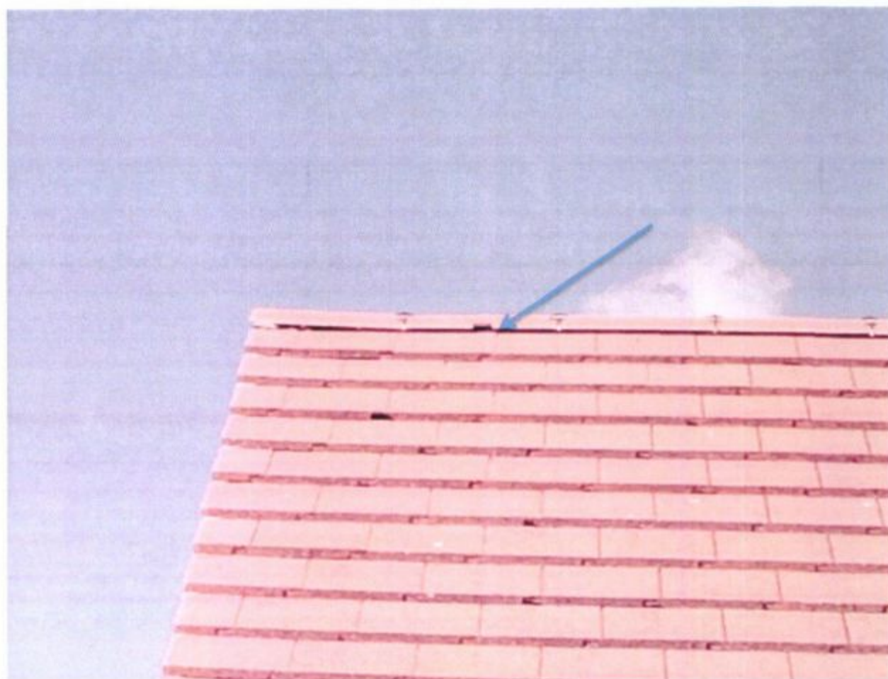
Gaps created around ridge tiles for bat access
