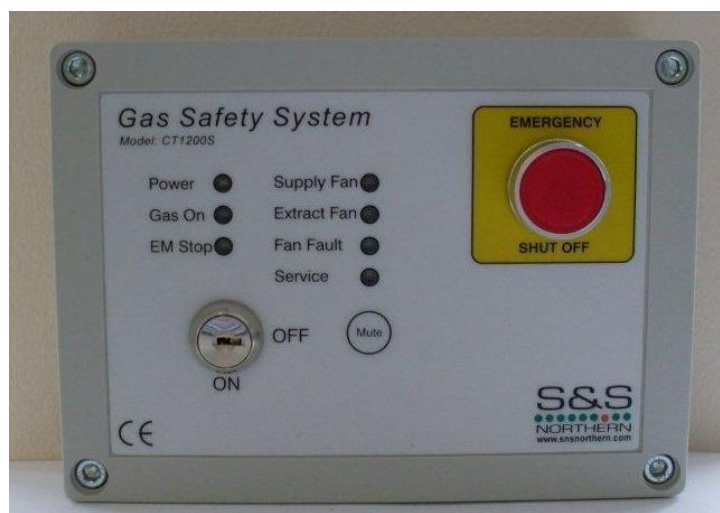
Fig 2 – Typical Gas Interlock Control Panel
