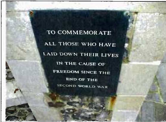
Generic plaque commemorating Post 1945 lives lost but also the rusting caused by incorrect fixings at the base of the plaque. This plaque would be replaced.
