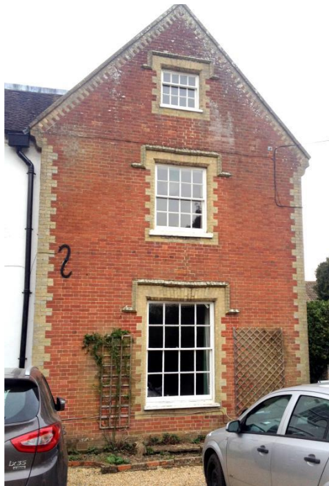
Fallen window arches on western aspect of south wing
