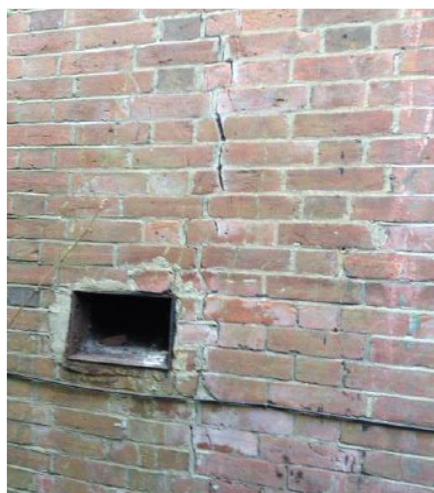
Crack to brickwork on southern aspect of south wing.
