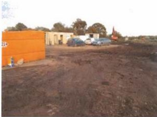
Photographs showing the clearance of the area of waste oil spillage
