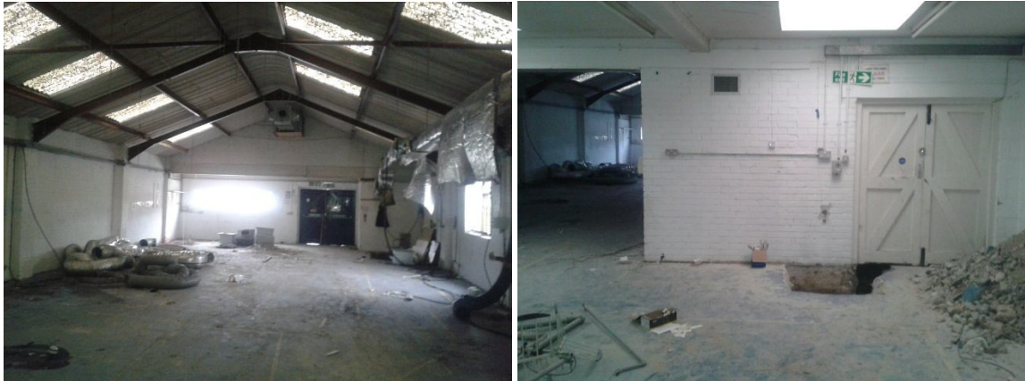
Images #4&5 – Views inside the old print works, with asbestos cement roofing, steel framed building style & recent electrical safety works issues all in view.
