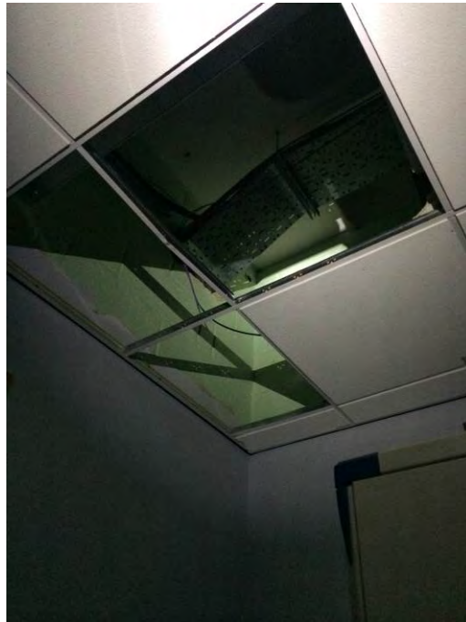
Photograph 13 – Missing ceiling tiles
