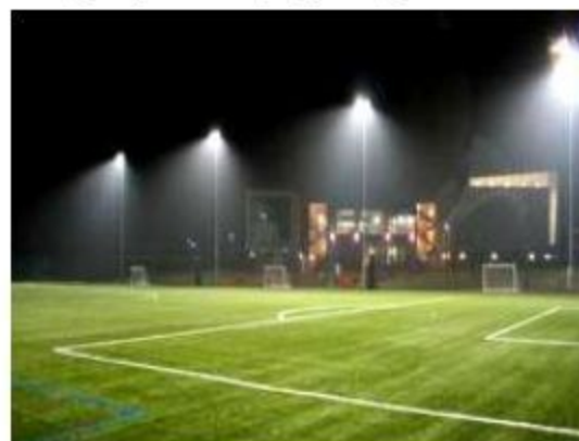
Example of floodlighting
