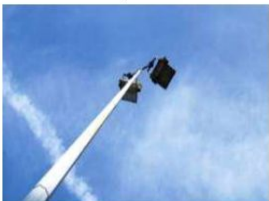
Example of 12m high floodlight
