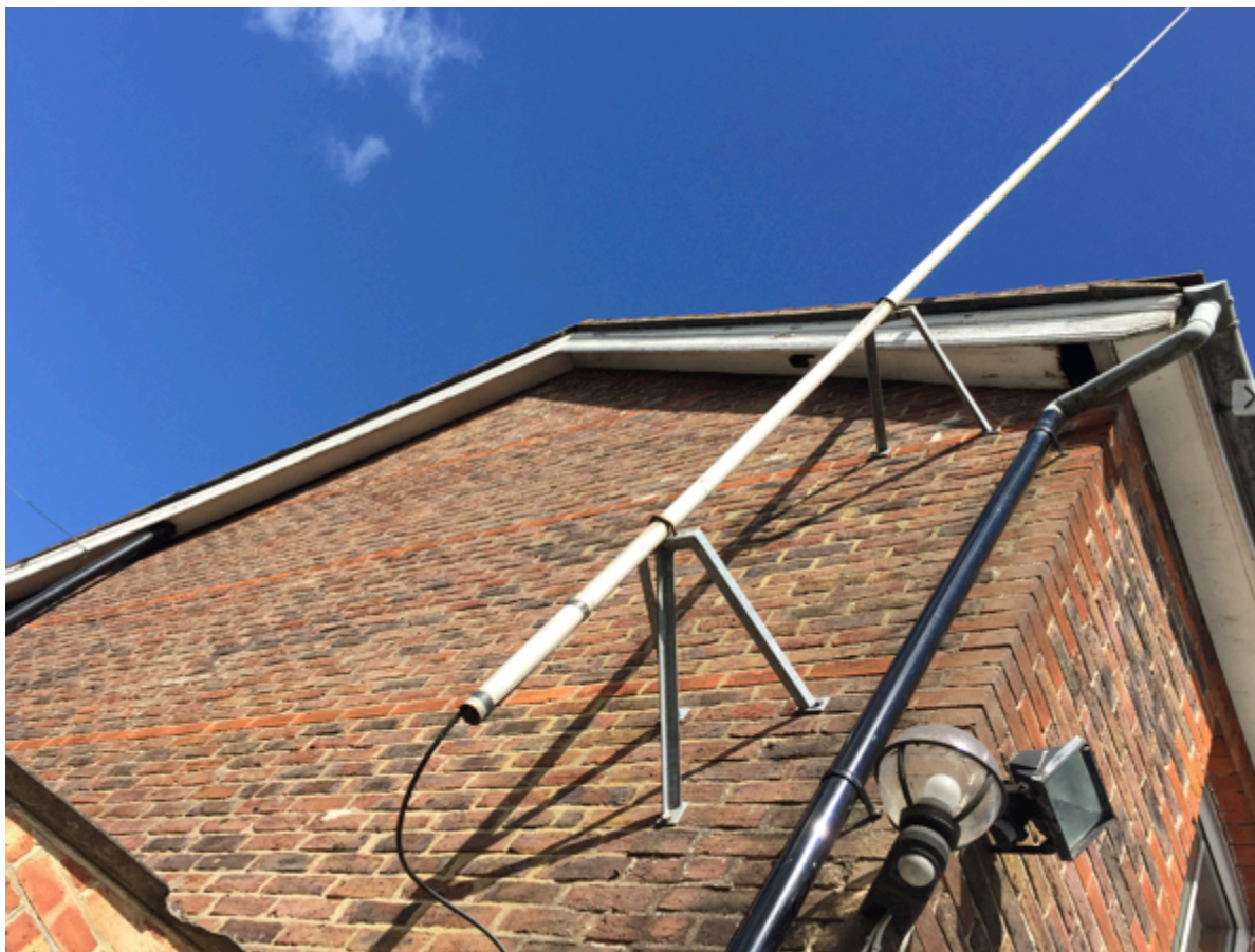
Figure 4. The section of rotten soffit boarding at the gable end of the roof, offering some potential for access by roosting bats.
