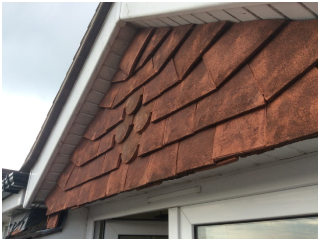
Figure 4. The tight fitting PVC soffits devoid of potential bat roosting gaps upon the eastern elevation of 40 Bath Road.
