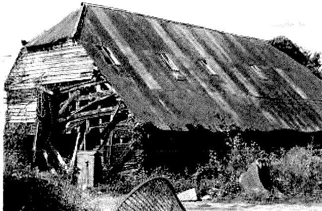
Antrims Barn was in a very dilapidated state in 2011.
