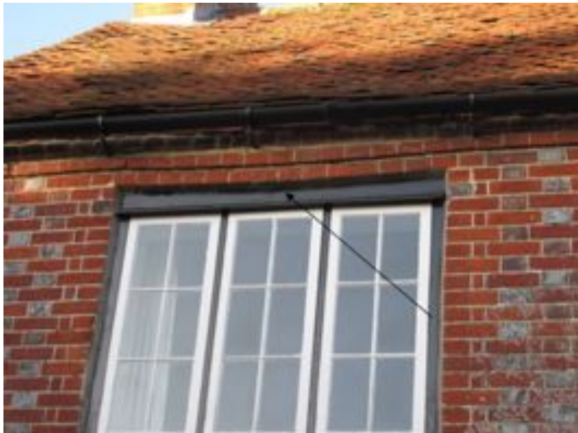
Fallen brickwork over window head
