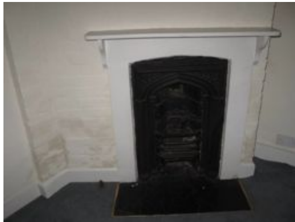
The damp fireplace wall
